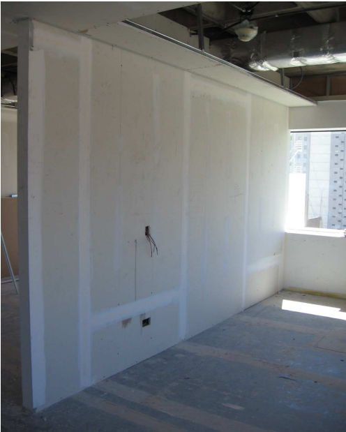
MANAGER'S OFFICES - DRY WALLS AND CEILINGS - METAL STRUCTURE + GYPSUM BOARD + ACRYLIC WALL PUTTY
