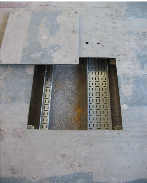
OPEN SPACE - CABLE TRAYS UNDER TECHNICAL FLOOR
