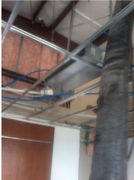
AC new unit in coffee area
